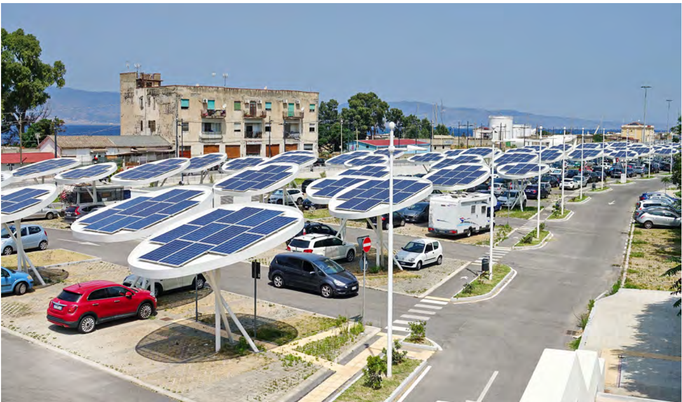
Solar panels in a car park. Companies are installing renewable energy sources to reduce their carbon footprint. Reggio Calabria, Italy
