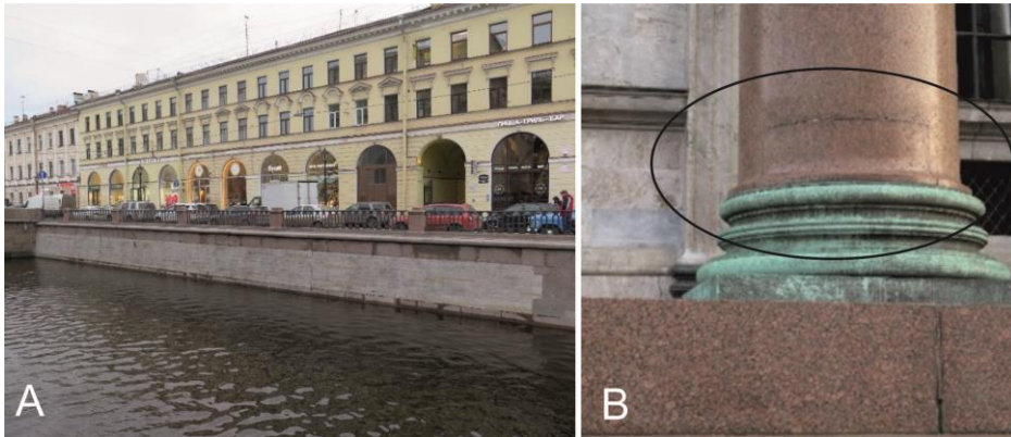
Figure 5. A. Channel embankment, in the centre of the embankment is visible the substitution of original material, rapakivi granite, with different stone type, limestone. Photo: Heikki Pirinen. B. Restoration of the lower part of pillar using same rock type as original at Cathedral of St Isaac. Photo: Mika Räsänen.
