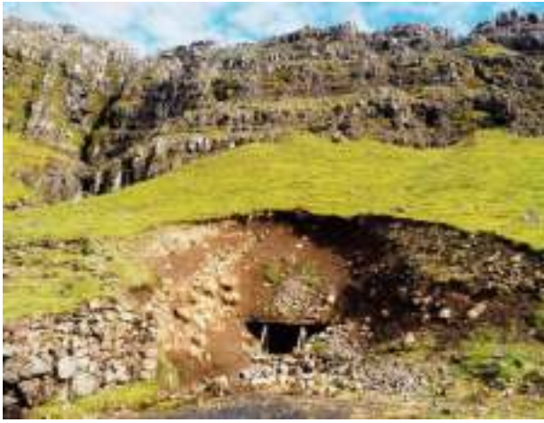
Figure 3: Abandoned mine of “Rókhagi” – a large slide of basalt blocks around the adit portal.
