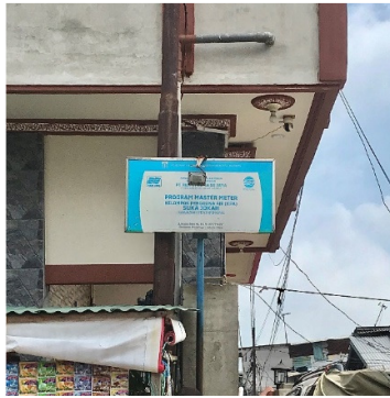
Fig. 2: Signet Master Meter in Kembang Lestari Village, Penjaringan, North Jakarta.
