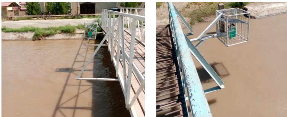
Fig. 21. Smart devices for determining water flow installed on the irrigation canals.
