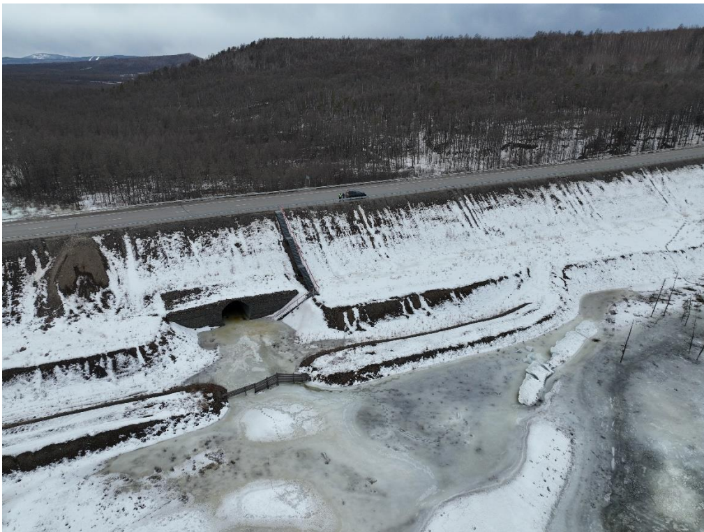
Figure 1. Icing phenomena along the “Lena” highway and anti-Icing facility on the Banniy creek
