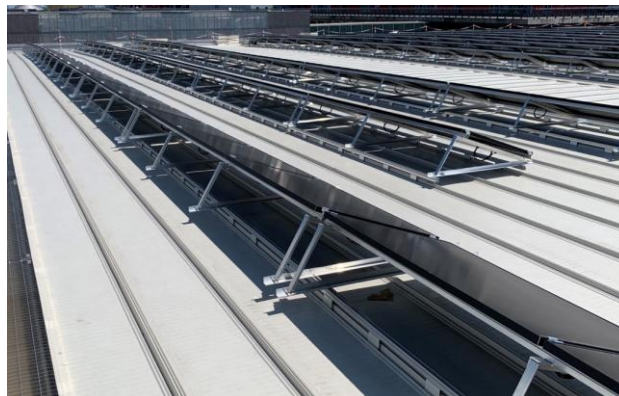
Figure 5. Example of tilted PV strings attached onto a flat standing seam roof.
