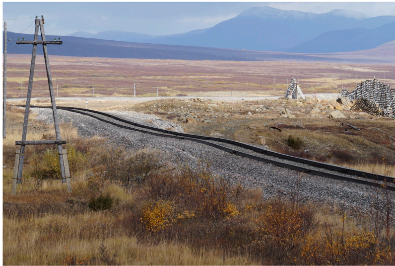
FIGURE 2 | Railroad deformation associated with permafrost degradation along the North Russian Railway close to the Khanovey field site at the western foothills of the Ural Mountains.
